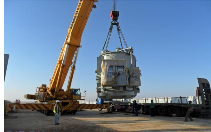
Transformers – 76 tons, 144 cbm, 24 pieces
